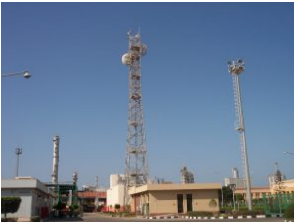
Petrobel 48m radio tower - Elgamil site
